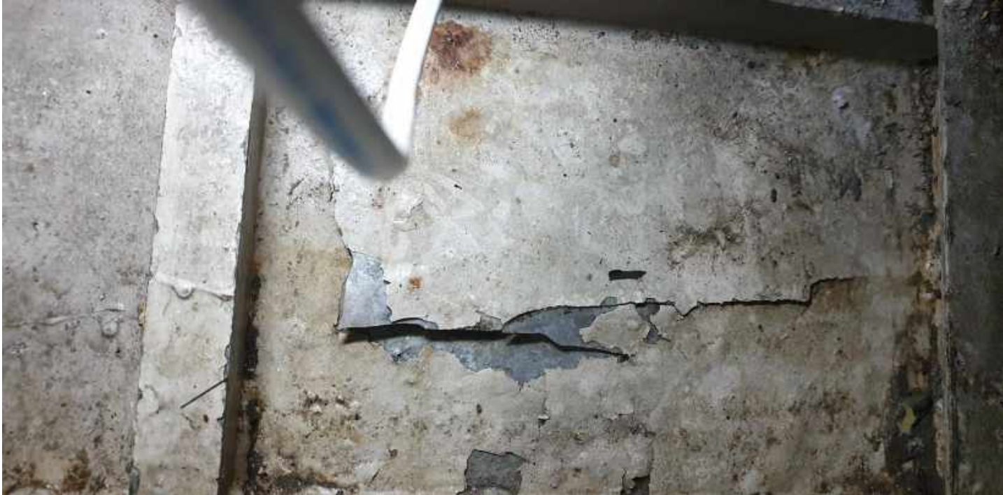
Picture of crack in Hull from inside prior to Temp Repair taken in Sept 2019.. supplied by Client
